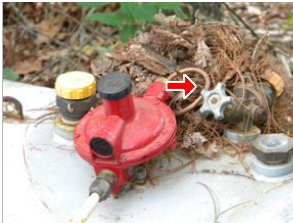
5.5 Picture 1 Propane Tank
