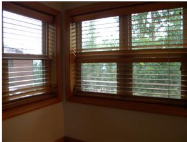
1.2 Picture 1 Tight operation of windows - master bath
