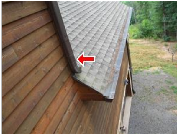
1.4 Picture 1 Gutter empties to roof
