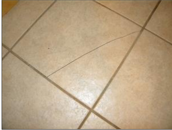
4.2 Picture 1 Tile crack
