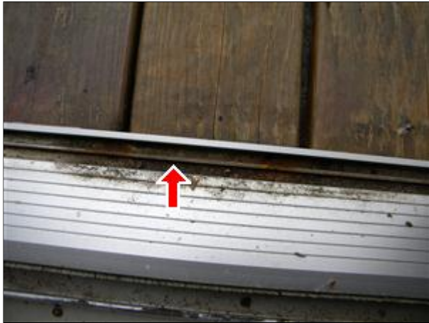
1.1 Picture 1 Minor Rust
