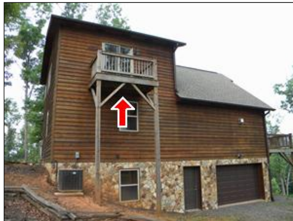
1.3 Picture 3 Ledger lacks bolts
